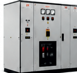
7. VCB HT PANEL
